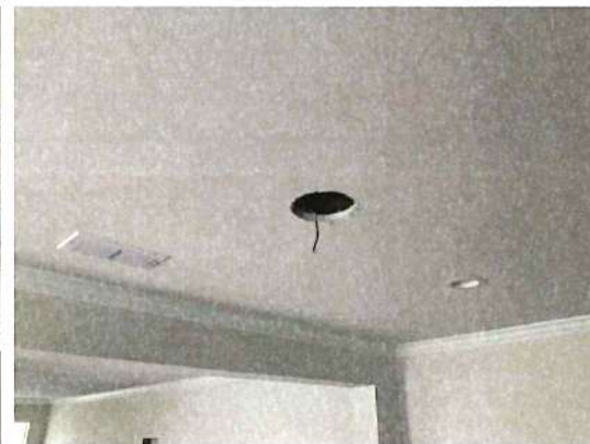
Dining - Hole in Ceiling for A/V
