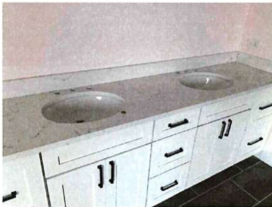
Bath - Hardware Not Installed
