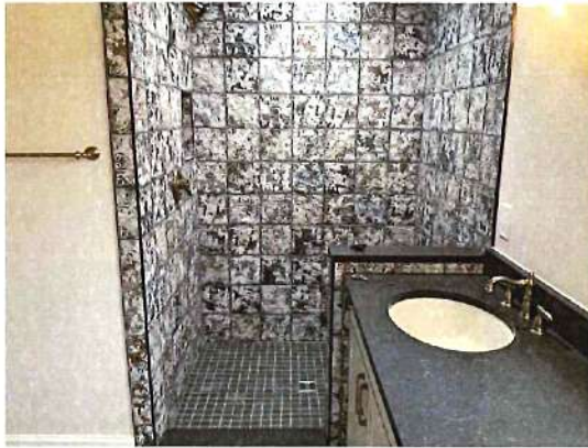
Bath - Shower Glass Not Installed - Not Required But Market Expected For a Shower Like This.
