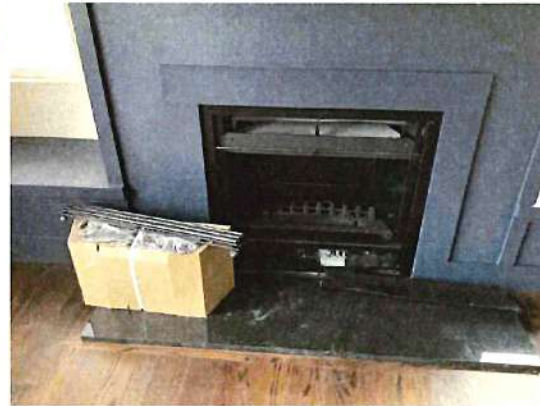
Family - Fireplace Hardware Does Not Appear to Be Fully Installed
