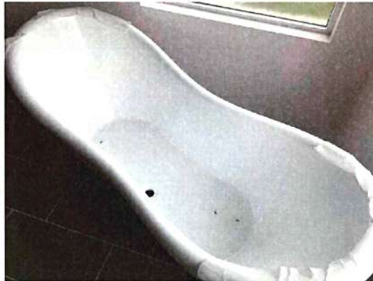
Bath - Tub Not Installed - No Hardware
