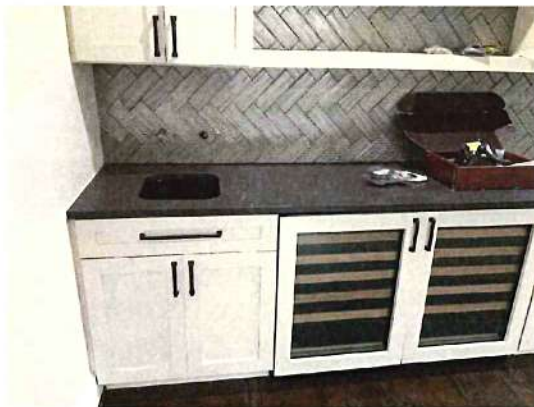
Wet Bar - Hardware at Sink Not Installed
