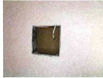
Missing TV Bracket
