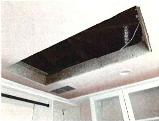
Closet - Drop Stair Not Installed
