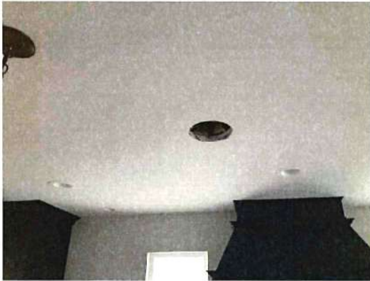
Kitchen - Speaker Missing - Hole in Ceiling
