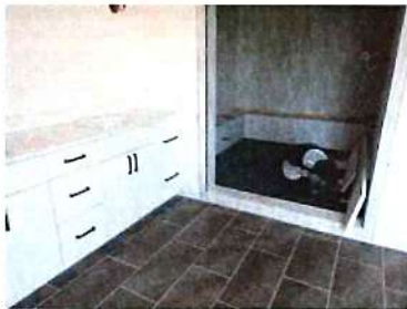
Bath (missing fixtures)
