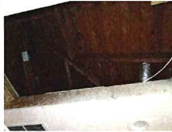
Missing attic cover
