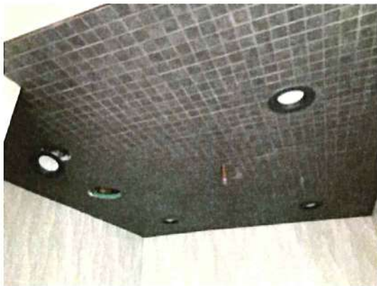
Bath - Main Shower Not Complete
