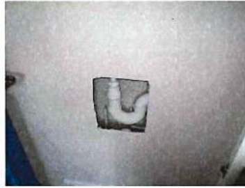
Example of repair needed
